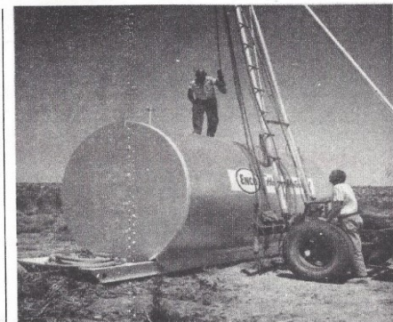
THOSE BIG DIESELS GULP A LOT OF FUEL SO AN 8000 GALLON DIESEL TANK WAS PROVIDED.
